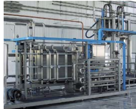
Aseptic Filling Unit
